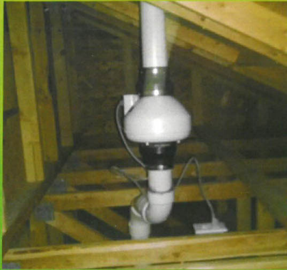
Radon fan installed in an attic.
